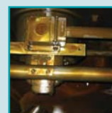
Varnish deposits (steering gear)
